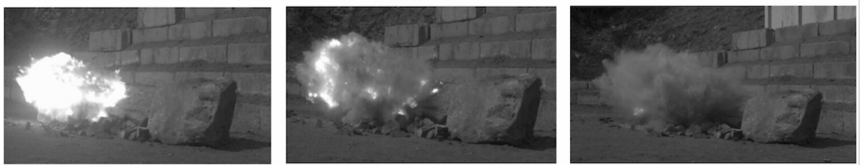
Top Left: Cone charges on boulders. Top Right: Post blast fragmentation results. Bottom: High-speed imaging of a boulder and cone detonation.
